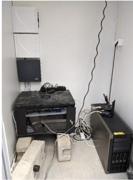
Figure 18. The server installed in an office container.
